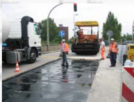
Deck surfacing with reaction resin filled porous asphalt Seaport bridge Hamburg Germany
